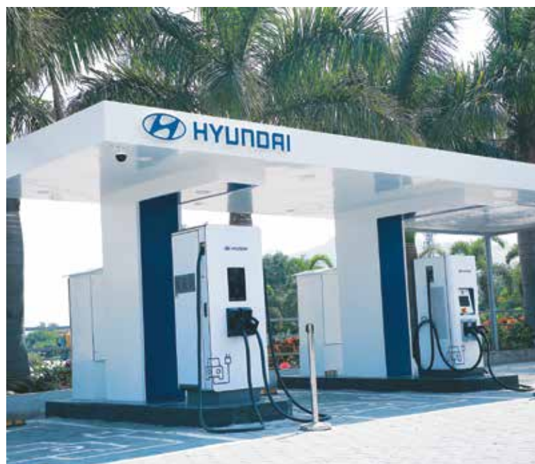
Hyundai DC charging station
